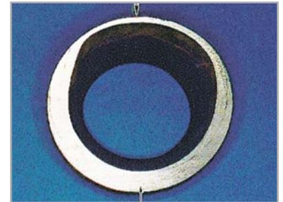
Internal wall thinning in a pipe subject to flow accelerated corrosion.
