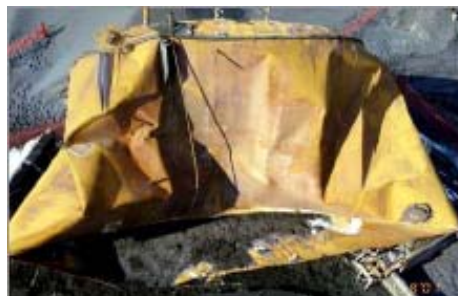
Collapsed Storage Tank.
